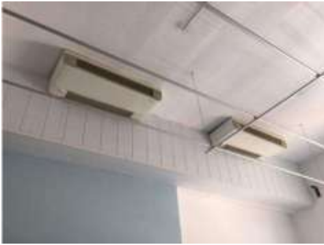
Fig. 12. Air conditioning of A18 classroom showcases an outdated Air conditioning model (taken by author)
