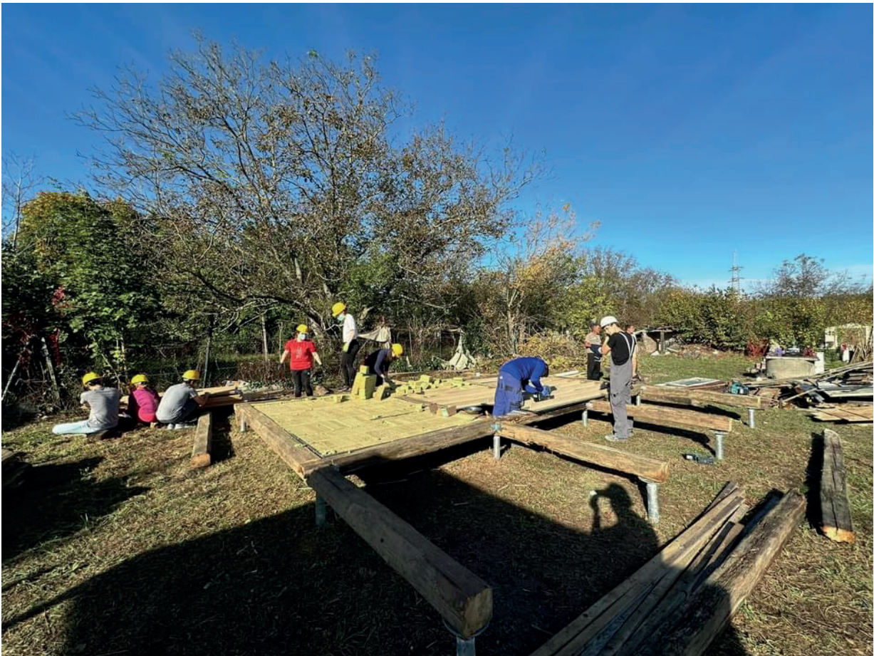
Fig. 3. The framework of the new building was made from old roof timber, lifted from the ground and attached to soil screws. The space between the beams were filled with leftover thermal insulation.
