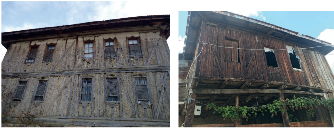
Fig. 4. (a) Adobe filling technique between wooden frame (Medinegil house); (b) timber infill wall between timber frame (Camadan house)
