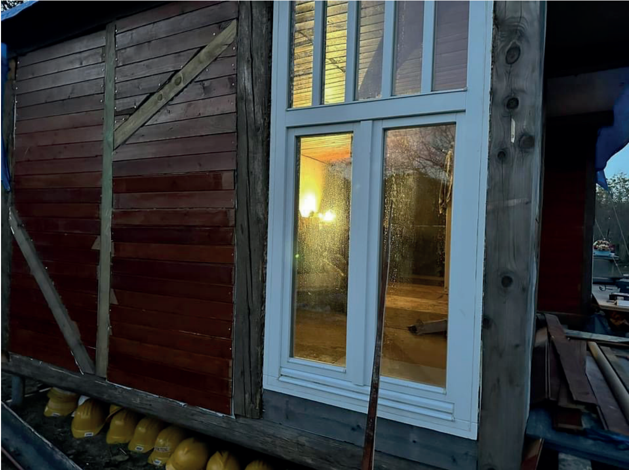
Fig. 4. Fachwerk framework filled with reused wainscoting and heat insulation. The window came from a hotel under refurbishment.
