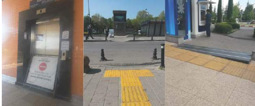
Fig. 5. (a) elevators under maintenance; (b) discontinuity on tactile paving; (c) difference of level
