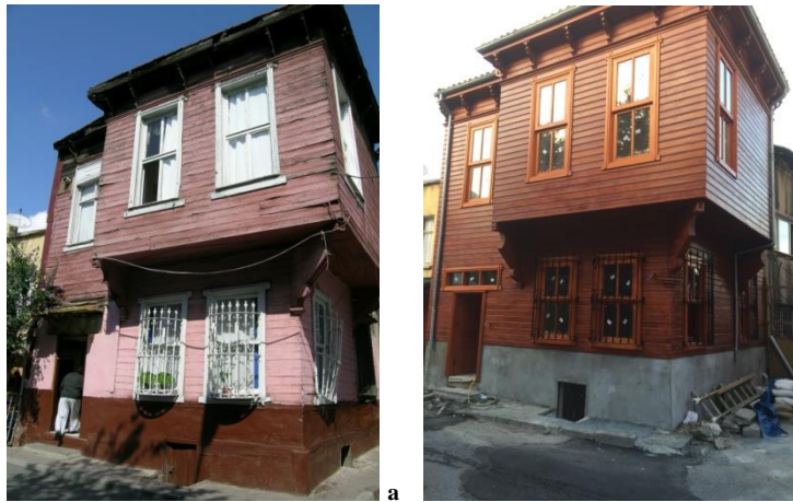
-Fig. 10. Badly restored example of civil architecture on the corner of Mustafa Pasha Bostanı Street and Mustafa Pasha Bostanı dead-end; a. before (Esmer, 16.09.2009) and b. after (Esmer, 05.10.2015) the restoration.
